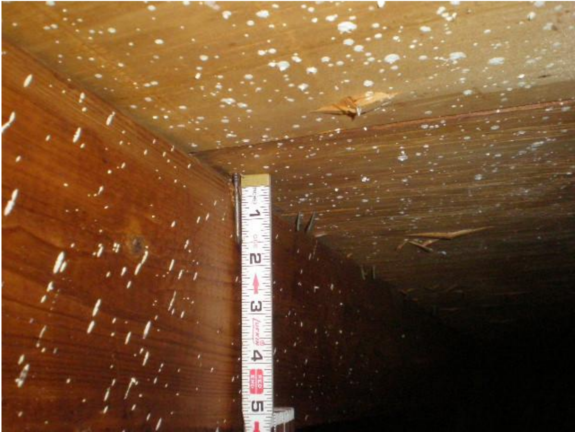
Roof deck 6d nails
