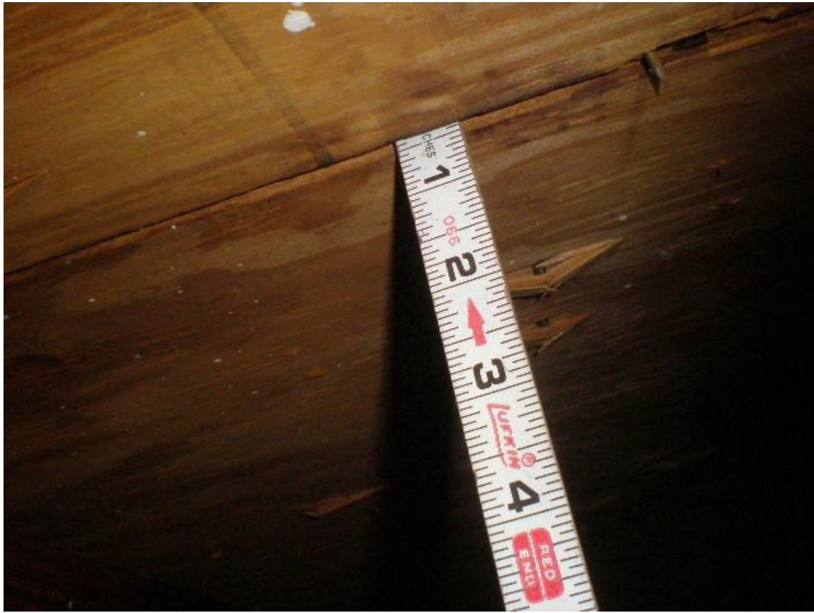
Roof deck 6d nails
