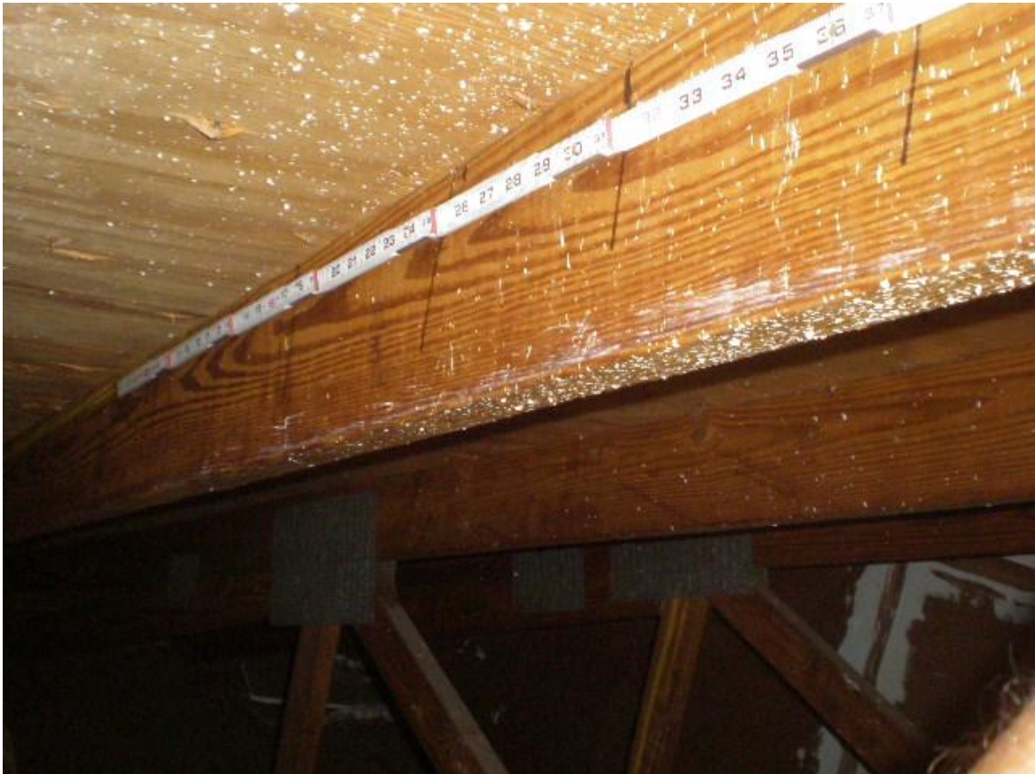
Roof deck 6d nails
